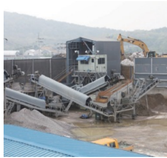
Conveying raw materials in cement factory
