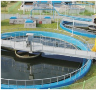
Aeration in sewage treatment plant
